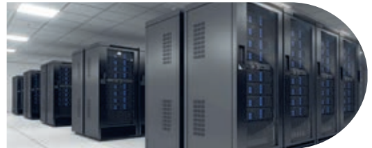
LARGE DATA CENTRE
