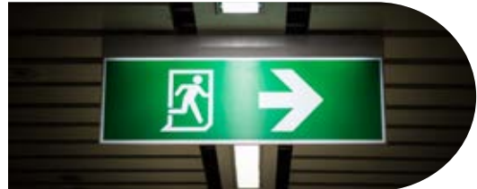
EMERGENCY AND SAFETY SYSTEMS
