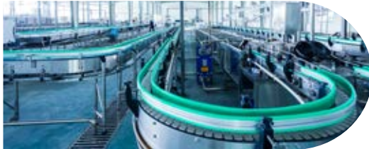
INDUSTRIAL CONTROLS AND PROCESS AUTOMATION
